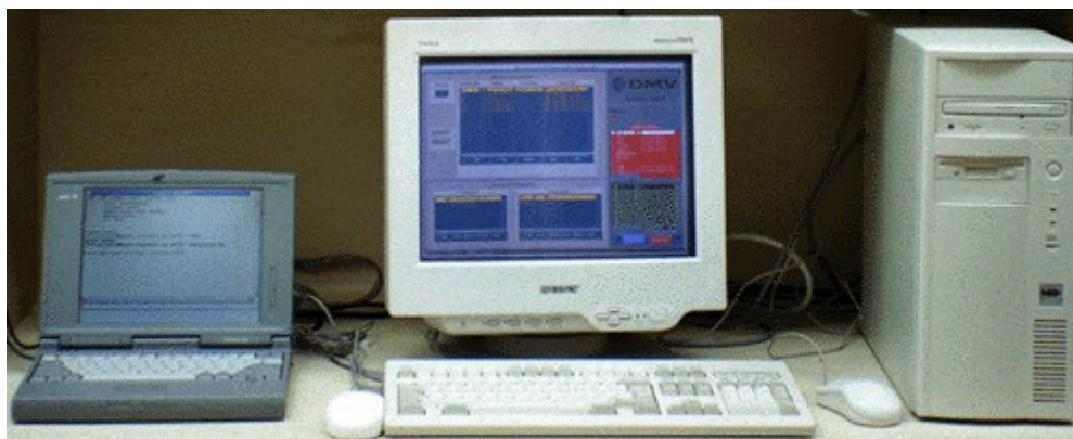
Picture 3 - Laptop for Modulator Control and MCC for Multiplex Control
